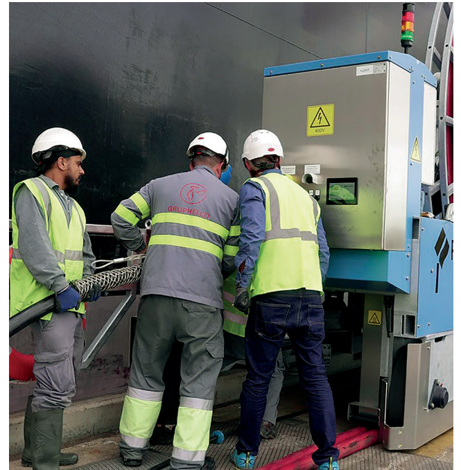
La terminal de Huchison Ports BEST es la única del Mediterráneo en poder conectar portacontenedores al OPS. / The Huchison Ports BEST terminal is the only one in the Mediterranean to be able to connect container ships to the OPS.
